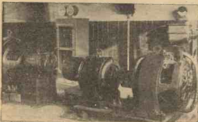
A view of the machinery room at the Dublin Station.
